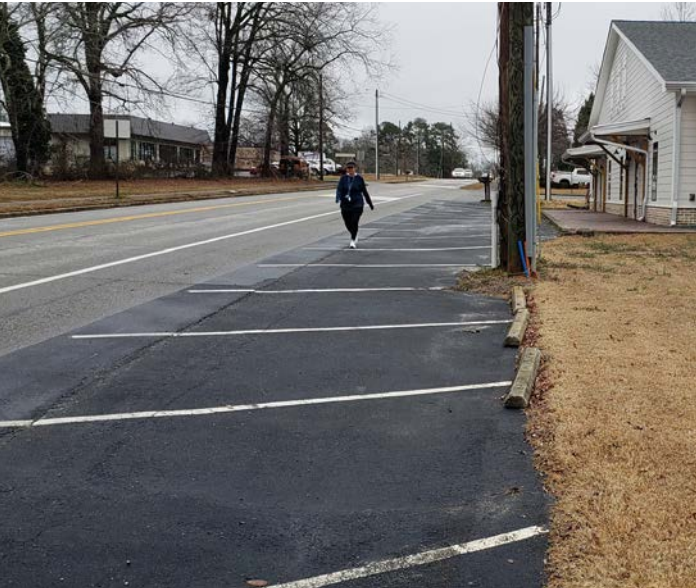
Sidewalks are interrupted in multiple locations
