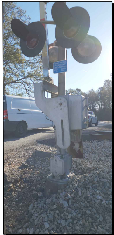
RAILROAD CROSSING ARM
