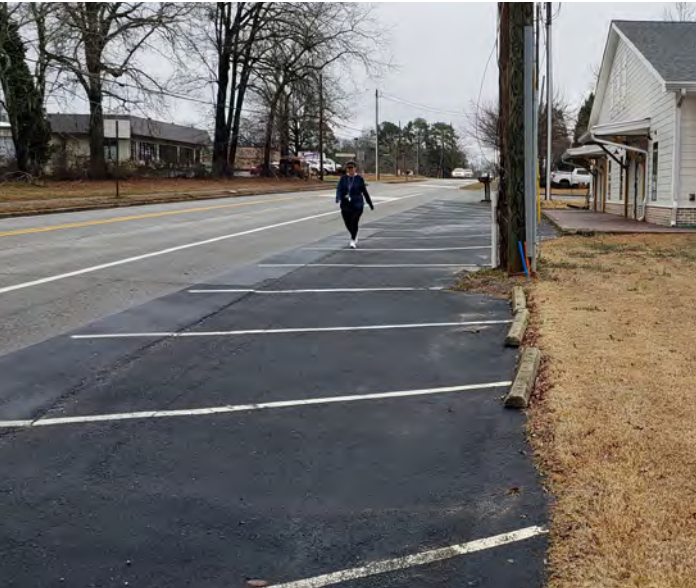
Sidewalks are interrupted in multiple locations
